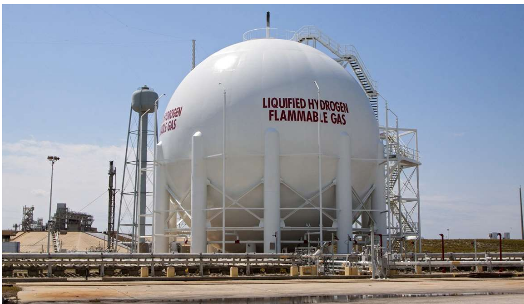
Figure 5-1 Hydrogen storage tank, Cape Canaveral (picture NASA)
