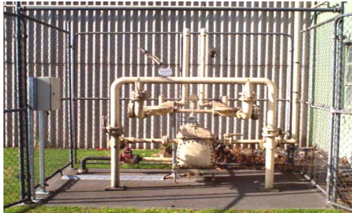
Figure 6 – Interval Meter (Large Gas Meter with Data Logger)
